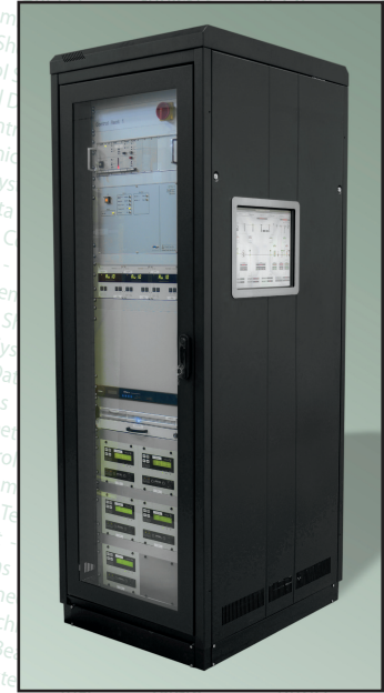
Beamline Control Rack with Touch Panel
